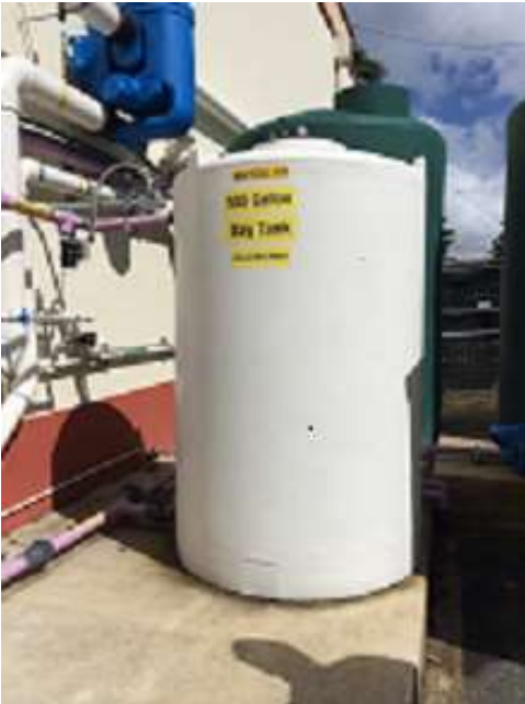
Rain Water Capture System, Fort Buchanan, PR ESPC
