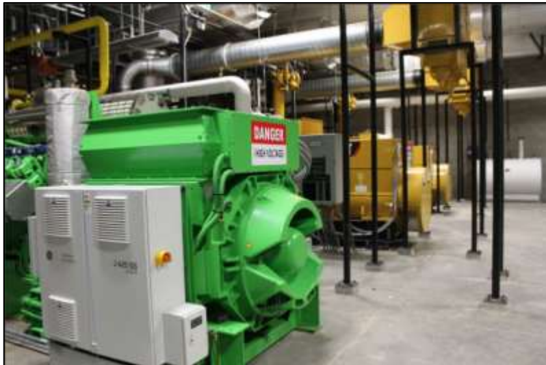
CHP Plant, Ft Knox
