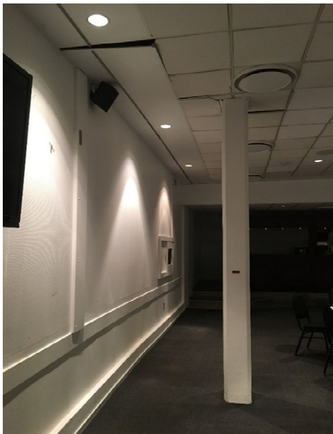
Figure 5-2. Left: A photo of a meeting room at a site in Thule, Greenland, where differential settling has led to wall and ceiling cracking. Photo by T. Douglas, CRREL.
