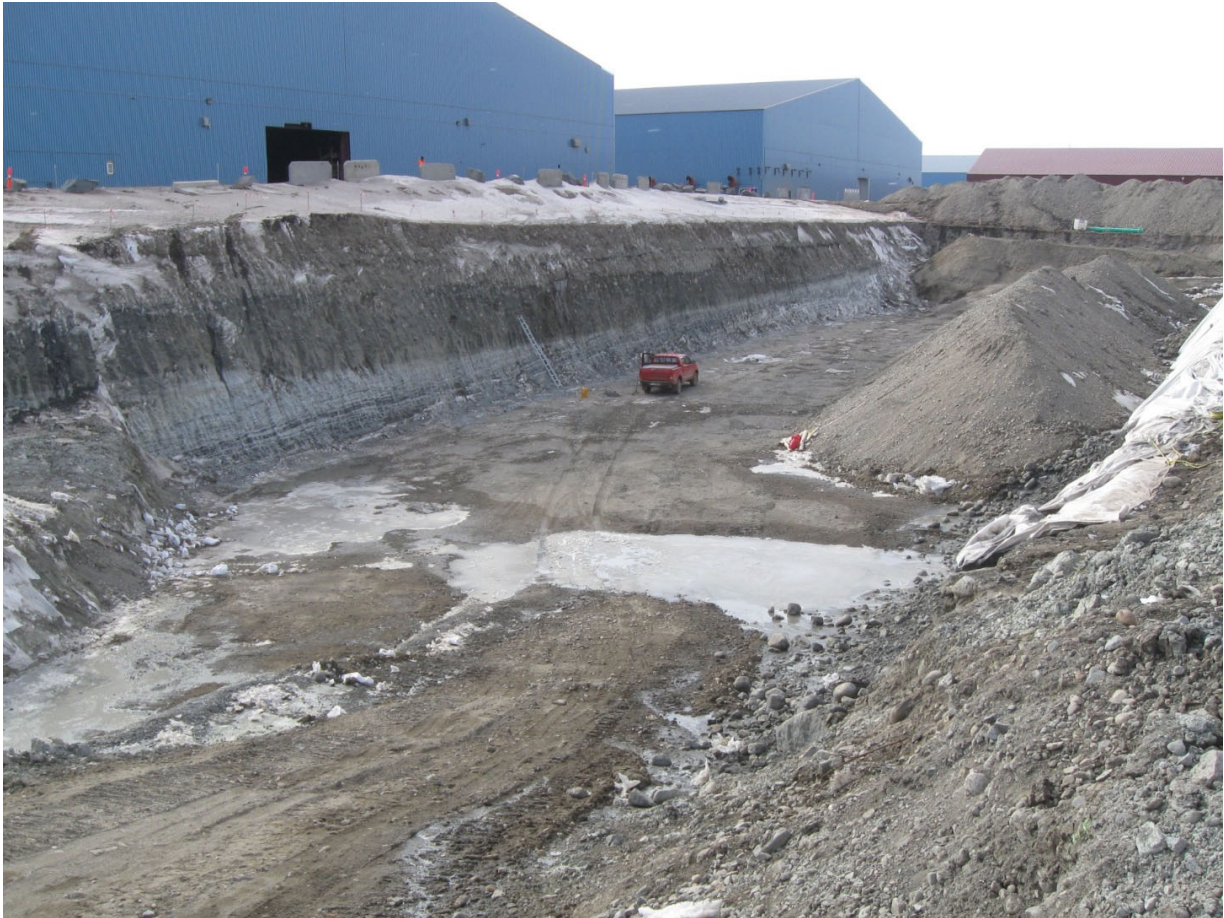
Figure 5-4. Removal of surface ice-rich permafrost and backfilling with thaw-stable materials allows for large slab on-grade construction. Photo by K. Bjella, CRREL.
