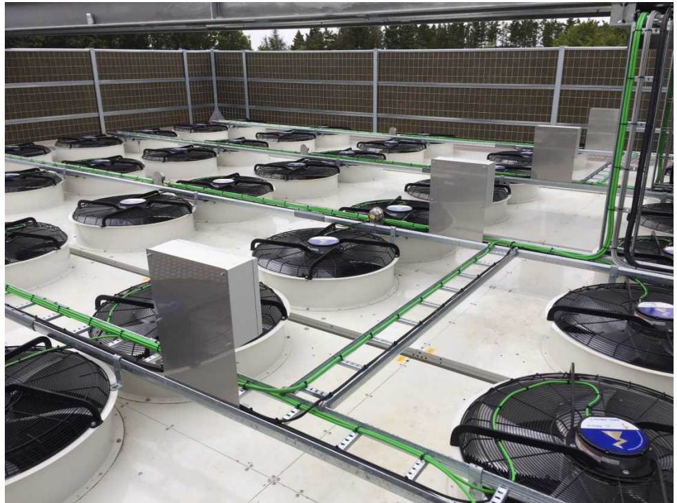
The intakes to the air-to-water heat pump system at Ringkøbing district heating plant.
