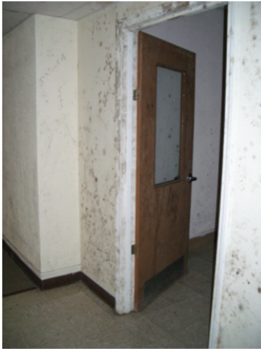
Figure 1-1 Mold growing on the surface of painted gypsum board and trim. Long-term high humidity is the source of the moisture that allowed the mold growth. All of the walls experienced similar near-condensation conditions. Consequently, the mold growth is widespread rather than concentrated in a single damp area.
