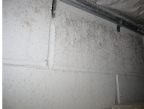
Figure 1-2 Mold growth on painted concrete masonry. The cool masonry wall separates a classroom from an ice rink. Humid air in the classroom provides moisture that condenses on the painted surface of the masonry. That moisture allows mold to grow on the paint film.
