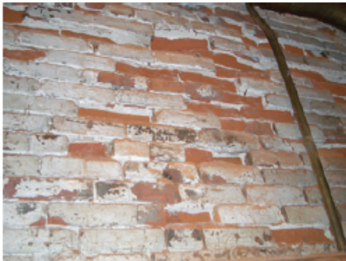
Figure 1-14 Damage to bricks caused by the migration of soluble salt through them. Salts in the brick or mortar dissolve in rainwater that wicks through the brick. The water evaporates in the building's interior, and the salt left behind crystallizes and splits the surface layer off the brick, exposing its interior. This process is called sub-fluorescence.
