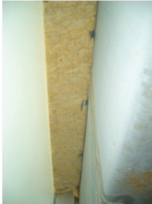
Figure 1-5 Corrosion of structural steel in a ceiling cavity in a cold climate. The steel extends into the exterior wall assembly. During cold weather, the steel near the wall is chilled by cold outdoor air. The building is humidified, and condensation from high indoor humidity provides the moisture that rusts the cold steel.
