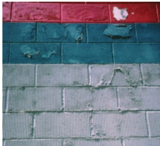
Figure 1-6 Blistering paint on split face concrete block. Wind-driven rain is the source of moisture contributing to the damage. Water wicks into the concrete masonry unit (CMU) through pin holes in the paint. The sun drives water vapor through the CMU. The assembly cannot dry to the interior because low-vapor-permeability foam board, taped at the joints, insulates the interior surface of the wall. The wall remains saturated throughout the spring, summer and fall. The same paint on areas of the wall sheltered from sun and rain shows no damage.
