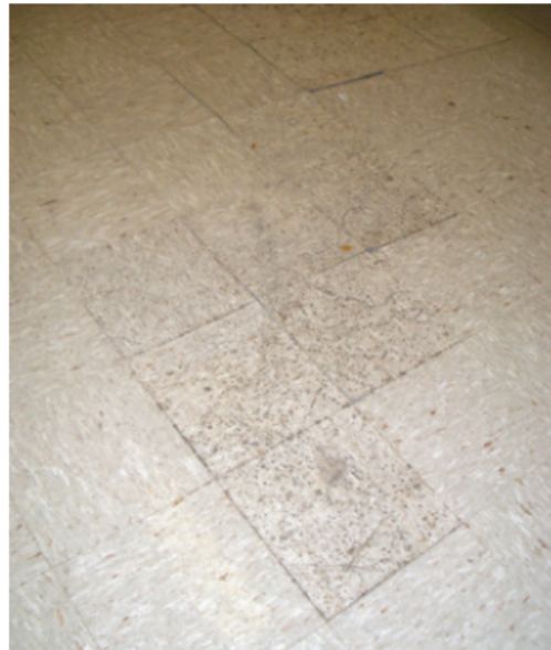
Figure 1-3 Mold growth on vinyl floor tile. Long-term high humidity provided moisture that was absorbed into the cool vinyl tile and supported mold growth. Also note that the high humidity caused the adhesive attaching the tile to the floor to fail, allowing the tile to become loose.
