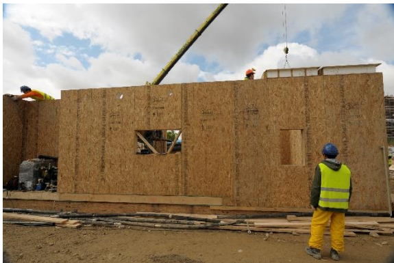
Figure 49: Construction of the 2010 TUC house on day nine of assembly at the SDE 2010 event site. Source: SDE, Flickr, Javier Alonso Huerta [sde flickr doc]
