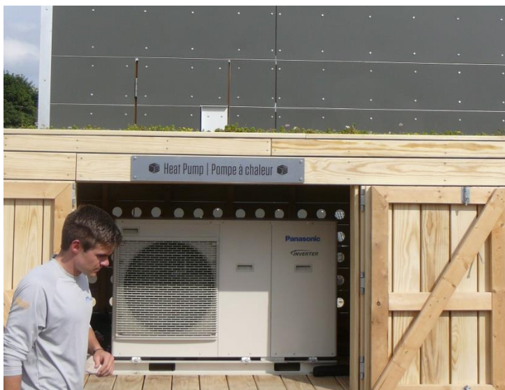
Figure 122: Split system compressor outside a building at SDE 2014. Source: University Wuppertal
