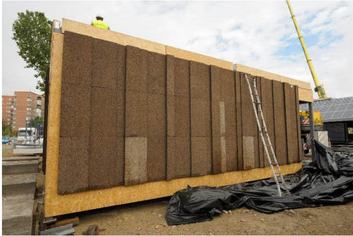
Figure 58: Cork insulating boards visible at SDE 2010 during assembly. Source: SDE, Flickr, Javier Alonso Huerta [sde flickr doc]
