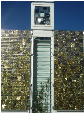
Figure 39: Solar chimney as part of the SDE 2010 HFT house. Source: University Wuppertal, Karsten Voss
