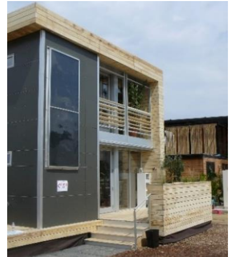
Figure 111: Façade-mounted flat plate collectors at a house at SDE 2014, Source: K. Voss, University Wuppertal
