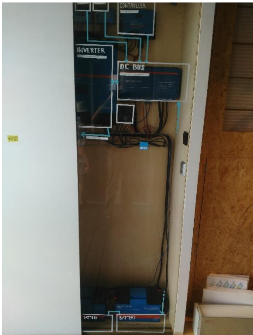
Figure 107: Small battery pack with lithium-ion technology as part of indoor house installation at the SD house of the MOR team in the SDE competition in 2019, Source: K. Voss, University Wuppertal
