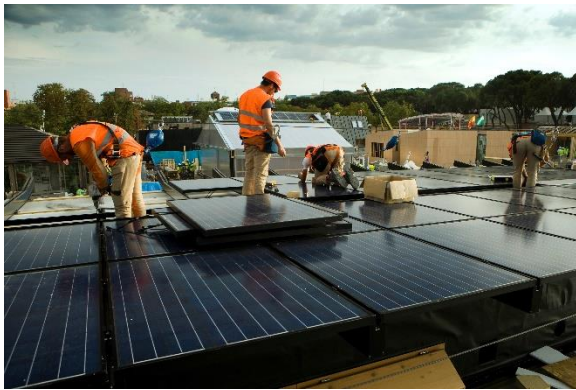
Figure 102: PVT hybrid modules form the roof of the Med in Italy house (ROME 2012). Source: SDE Flickr [sde flickr]
