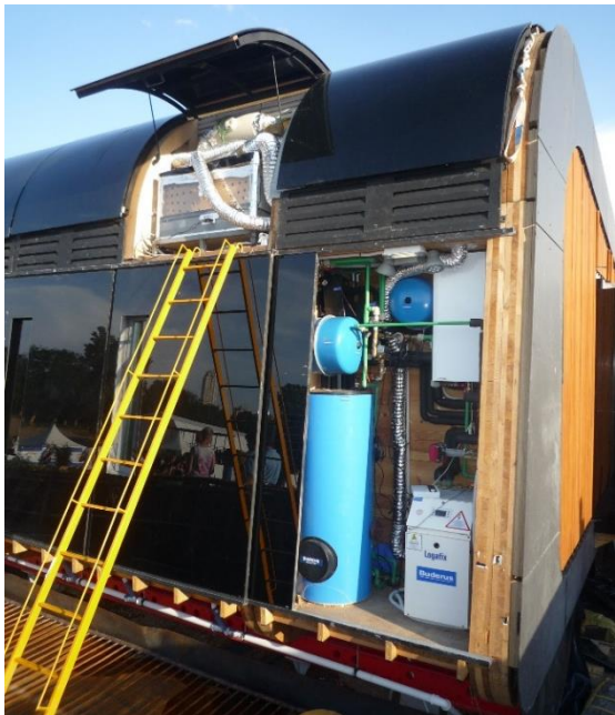
Figure 124: Service room with heat pump and thermal storage in an SDE house in 2010 in Madrid. Source: University Wuppertal
