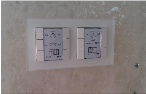
Figure 129: Typical low-voltage pushbuttons as part of the building automation system to replace classical switches for AC wiring (SDE 2012). Source: University Wuppertal
