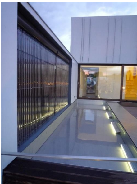
Figure 112: 6 m 2 vacuum tube collectors mounted vertically in an external wall of the BUW team home at SDE 2010 in Madrid. Source: K. Voss, University Wuppertal
