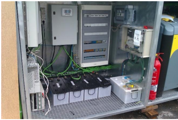
Figure 105: Four externally mounted batteries (bottom) with lead-acid technology at an SD house at SDE 2012, Source: K. Voss, University Wuppertal
