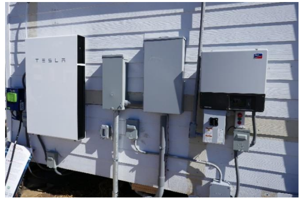
Figure 106: Externally mounted battery box (left-hand box) with lithium-ion technology at an SD house in the US competition in 2017. The capacity is listed at 13.5 kWh, Source: K. Voss, University Wuppertal
