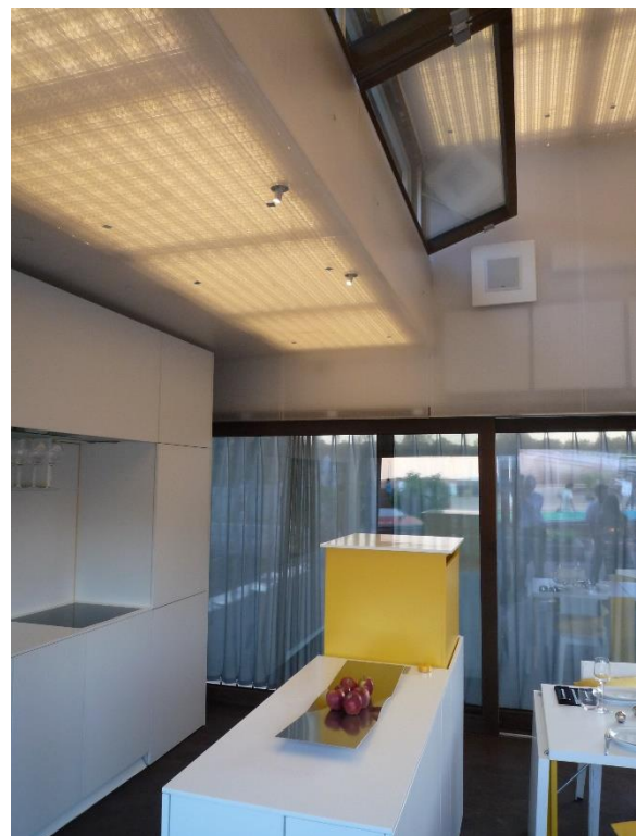
Figure 117: Energy-efficient lighting by LED systems within an acoustic ceiling and integrated movement sensing (SDE 2010). Source: University Wuppertal
