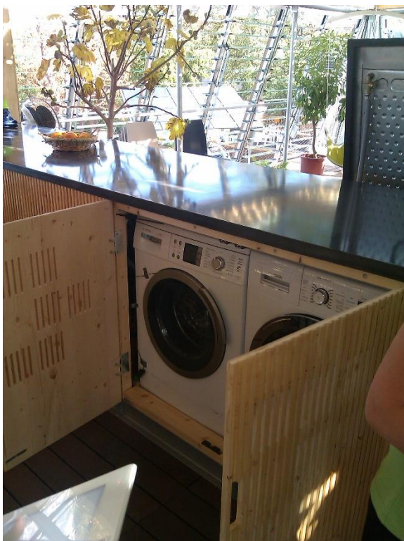
Figure 116: Example of the use of market available, energy-efficient appliances (SDE 2012). Source: University Wuppertal
