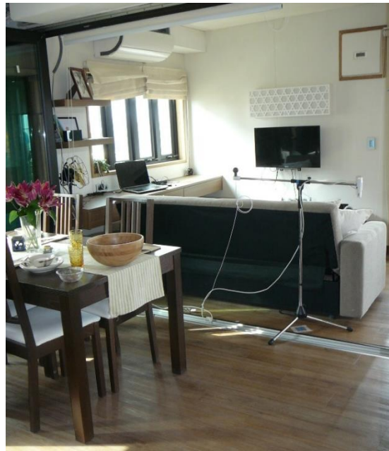
Figure 125: Visible installed ventilation components above the windows – internal components of a split system at SDE 2014. Source: University Wuppertal
