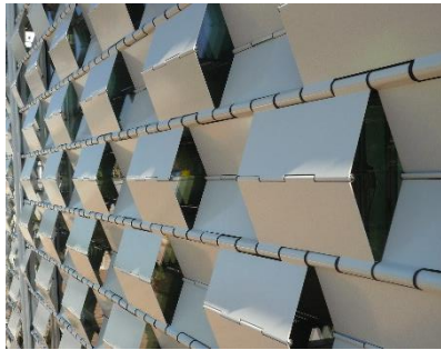
Figure 23: Moveable aluminum sun screen at the SDE 2010 ROS house. The profiles are specially folded to avoid direct light transmittance. The system as a whole is moveable from the bottom to the top and stored at the bottom of the façade. Source: University Wuppertal, Karsten Voss
