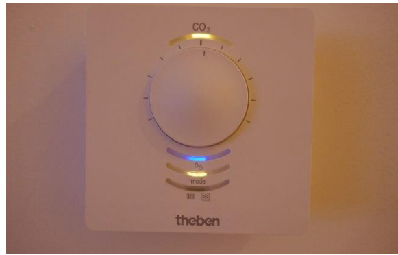
Figure 130: Turning knob to manually adjust the set point for a CO 2 -controlled ventilation system (SDME 2018). Source: University Wuppertal
