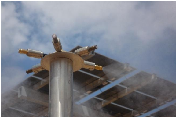
Figure 45: Evaporative cooling at the SDE 2010 site. Source: University Wuppertal
