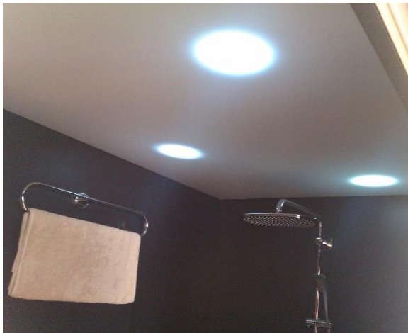
Figure 118: Daylight luminaires partly substitute artificial lighting in an internal bathroom (SDE 2012). Source: University Wuppertal
