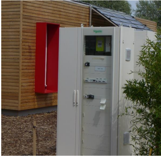
Figure 139: Typical grid access point at SDE 2014. Source: University Wuppertal
