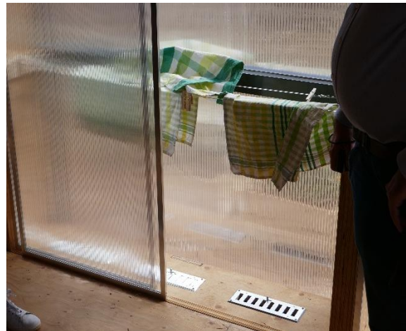
Figure 119: Integration of laundry drying in the circuit of the central ventilation system to substitute the operation of a dryer in the house of Team Lausanne at SD US 2017. Source: University Wuppertal
