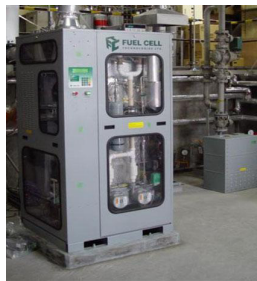
Figure 16: Stationary 5 kW (courtesy of Fuel Cell Technologies)
